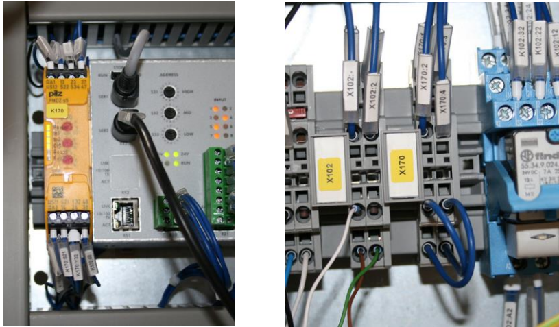
Fig. 3: Safety control device and terminals for safety device in the switch cabinet
