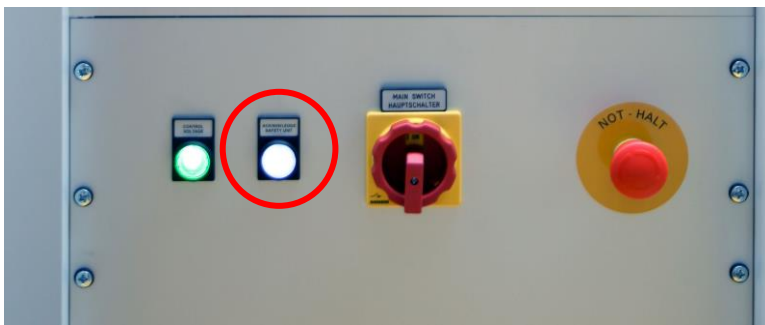
Fig. 4: Key for acknowledging the safety monitoring on the switch cabinet
